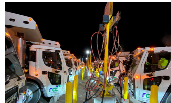
CNG Station Omaha, Nebraska (USA).
