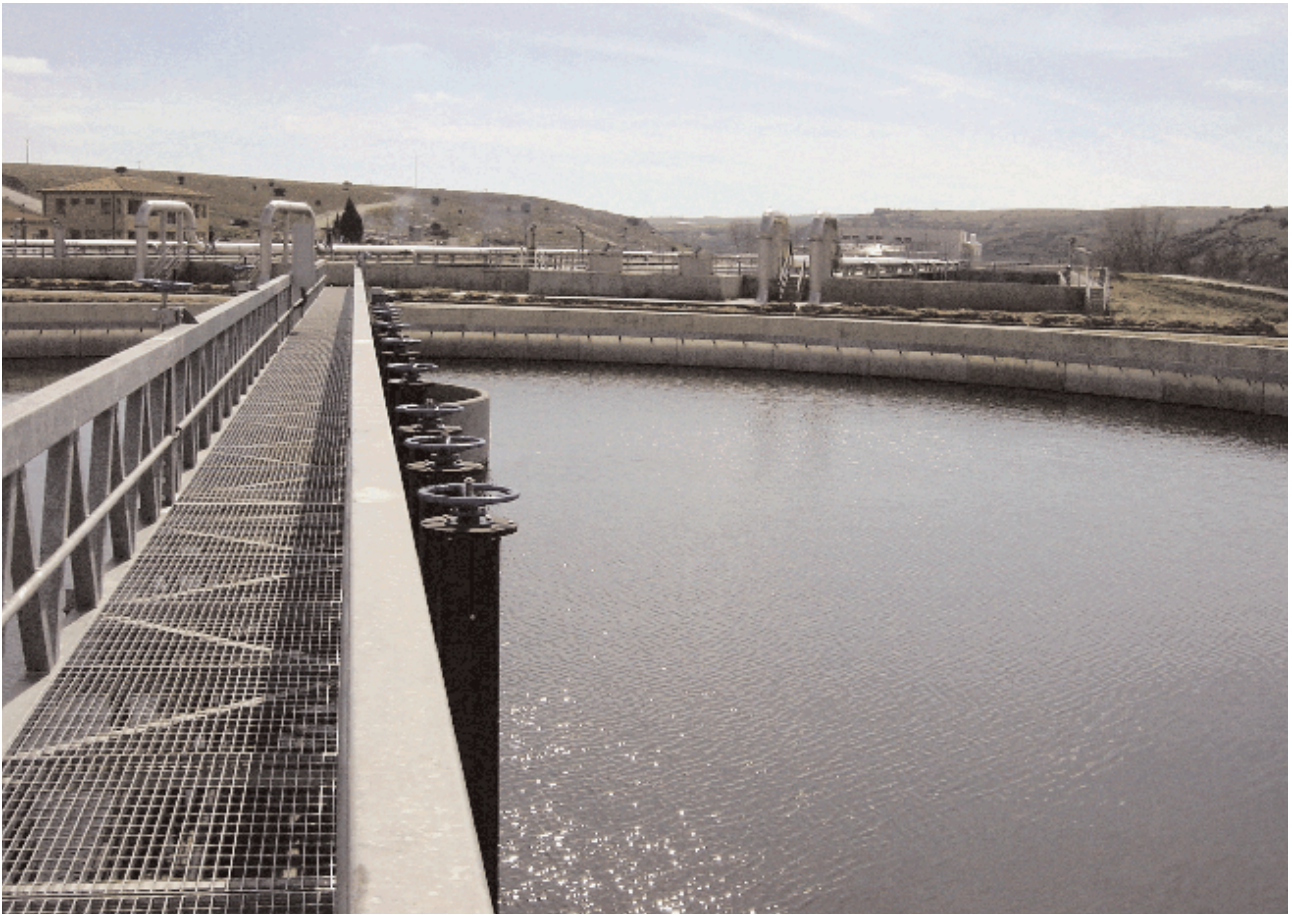
Wastewater purification plant. Salamanca
