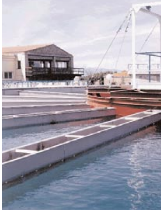
Drinking-water treatment station. Ávila
