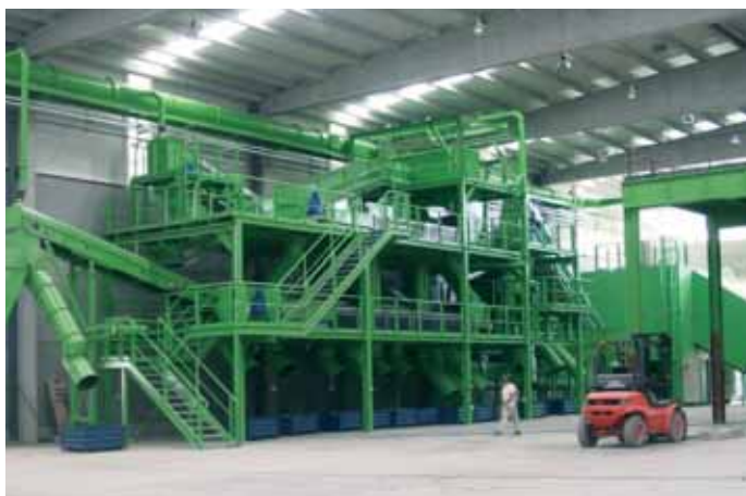
Recycling plant for refused electrical appliances and electronic devices. El Pont de Vilomara. Barcelona
