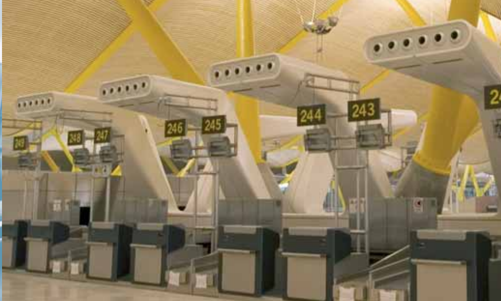
Central heating and cooling system for Terminal 4 at Madrid-Barajas Airport
