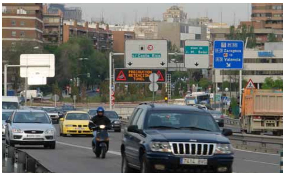
Remodelling work on the junction of calle Costa Rica with the M-30. Madrid
