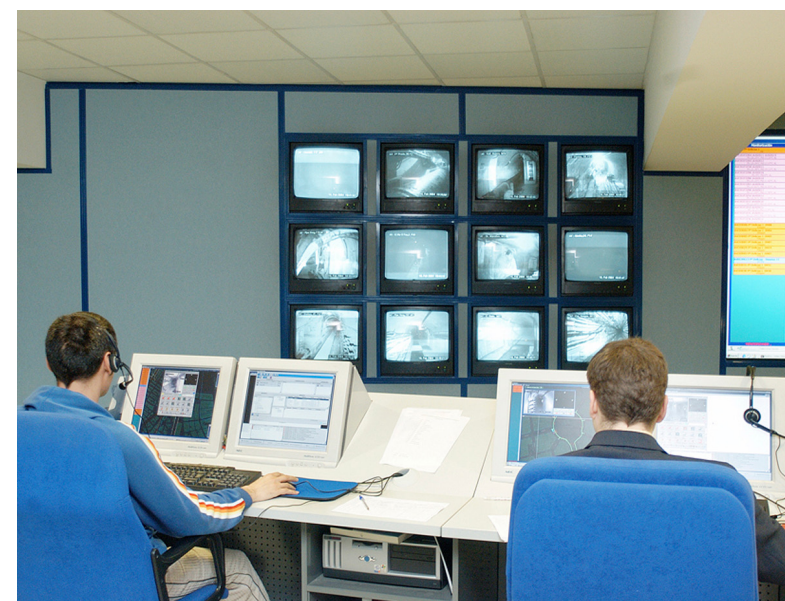
Control Center service tunnels, Madrid.
