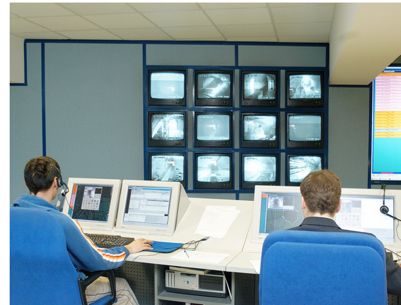
Control Center service tunnels, Madrid.
